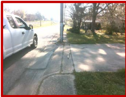
Power Pole Obstruction.
