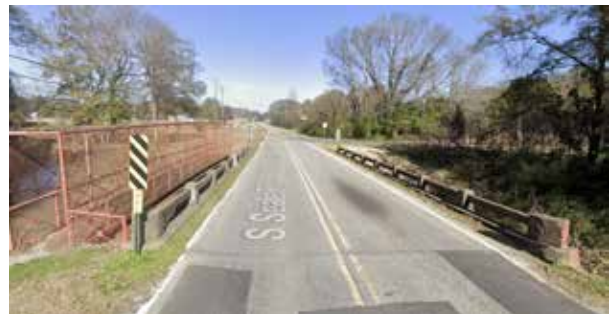
Existing Cochgalechee Creek bridge on Seale Road with sidewalk on west side
